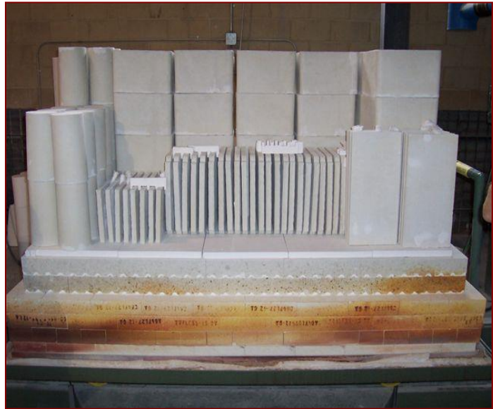
Recent Photo, No Maintenance
